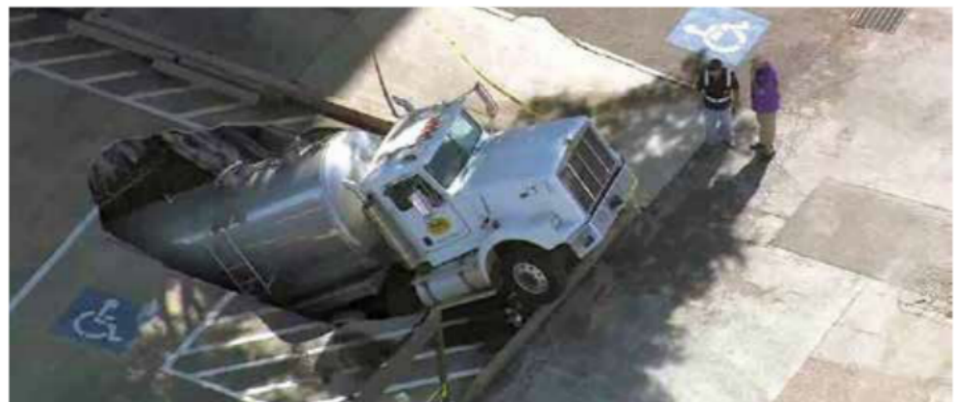
Deck failure, Houston, TX.
