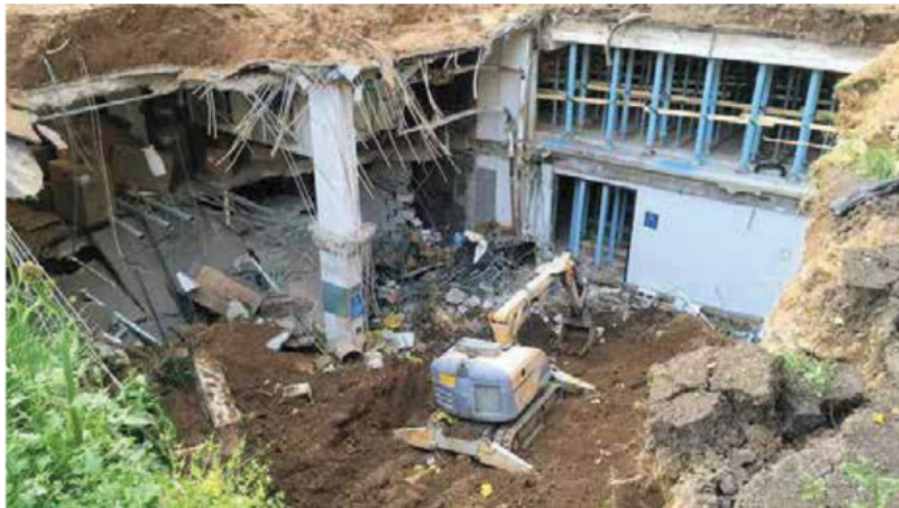
Garage collapse, Washington, D.C.
