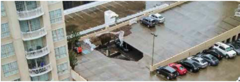
Pancake failure, Dallas, TX.
