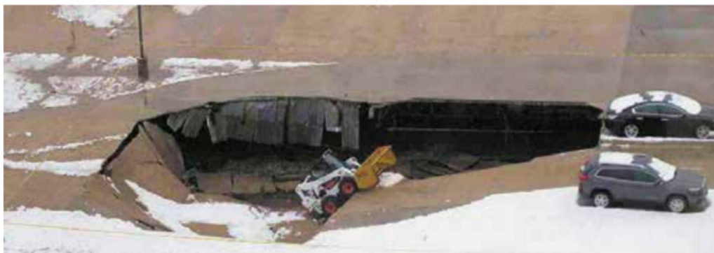
Failure caused by compacted snow pile, Secaucus, NJ.
